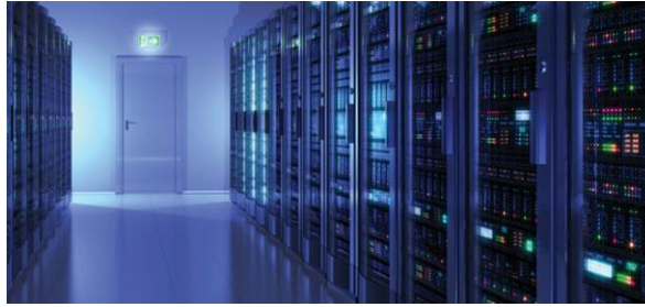
Data Center | Connectivity | FIBER
